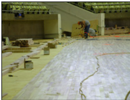
Workers have almost completed installation and look to paint the floor in the next few weeks.
